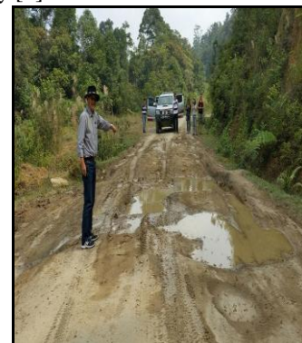
Figure 1.1: Example of the rural road condition in several areas in Sabah
