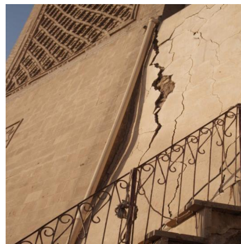
Fig. 2. Cracks appearing near the base of the minaret.
