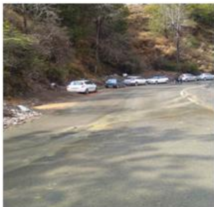
Fig.5. Poor Drainage condition (Near Shanan village)
