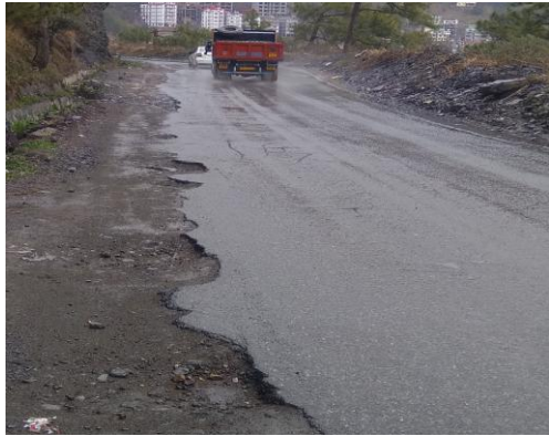
Fig.2. Detritions of the road edges (Near Malyana)
