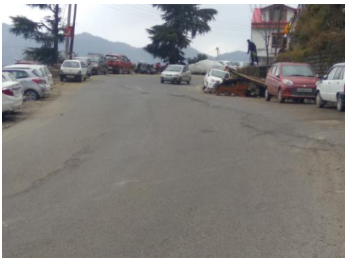
Fig.3. Settlement of the road because of poor compaction (Near Mehli)
