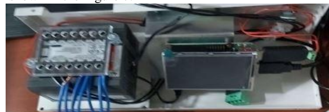
Figure 7: Smart Meter Connections
