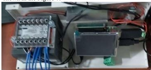
Figure 7: Smart Meter Connections
