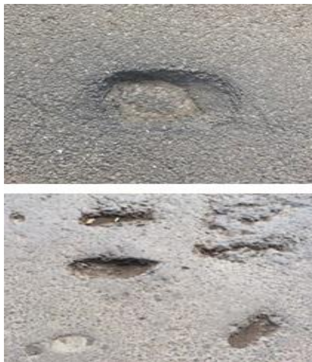
Fig. 1. Example of Potholes.
