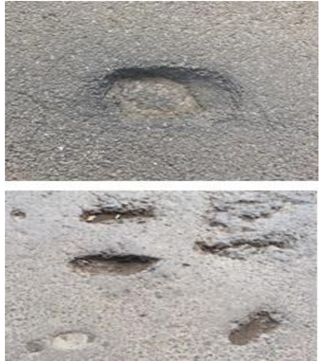
Fig. 1. Example of Potholes.
