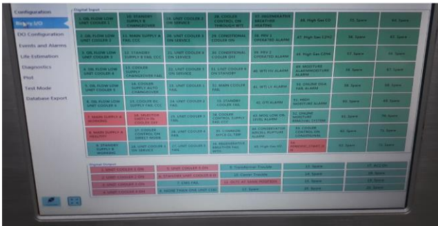
Fig. 5. Monitored Data at Control Room
