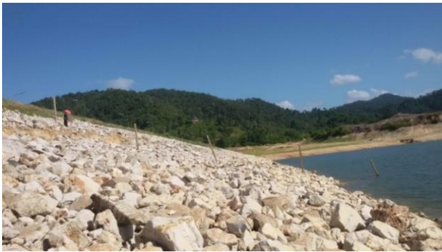
Fig. 2: Pa Bon dam after its movement on 14th January, 2004
