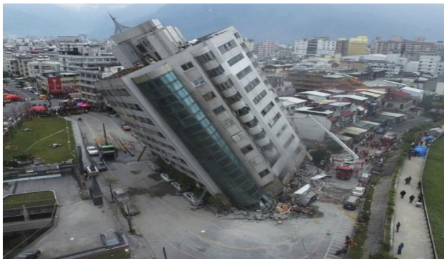
Fig 2: Differential settlement due to liquefaction
