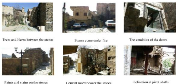
figure 12: the problems that have been detected in the stones of the village
