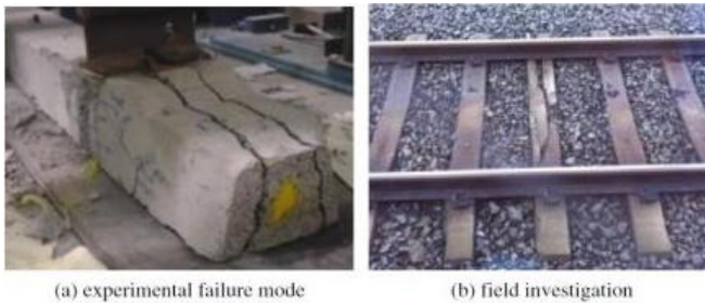
Fig. 13. Splitting failure caused by impact loading in concrete sleeper [26]
