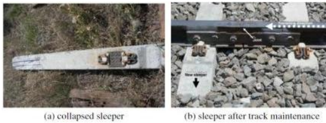
Fig.12. Impact damage due to rail irregularities to sleeper [30]
