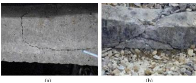
Fig. 14. Tensile fracture in concrete sleeper [32]
