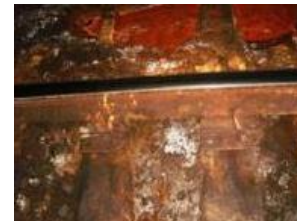
Fig. 21. Corrosion in steel sleeper [44].
