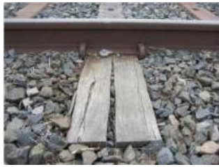
Fig. 3. Splitting at the ends (9)
