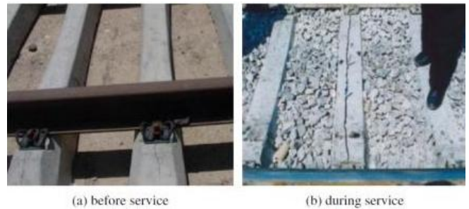
Fig. 15. Longitudinal cracking between rawlplugs [30].
