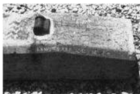
Fig. 20. Cracking due to DEF in pre-stressed concrete sleeper [41].
