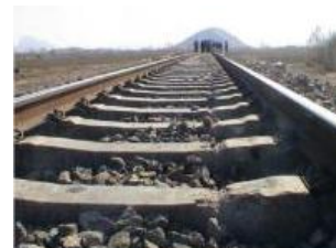
Fig. 10. Derailment of Concrete Sleepers [23]
