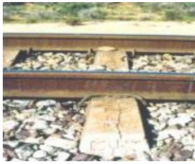
Fig. 18. Cracking due to AAR in concrete sleeper [38].
