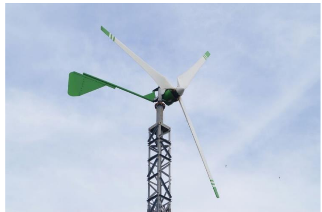
Figure 2. Wind power plant in Pantai Baru hybrid systems
