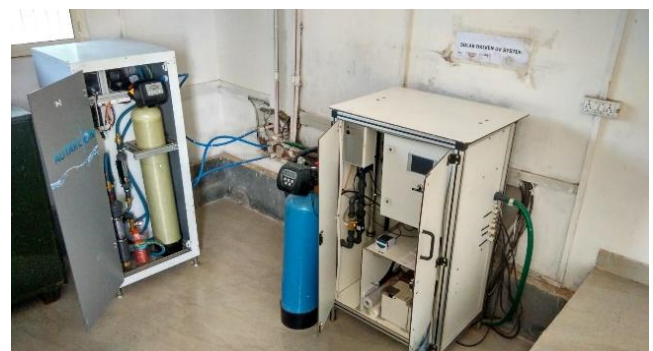
Fig. 2. Picture of AO & UV systems installed at SWINGS Pilot Plant AMU, Aligarh
