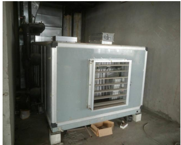
Fig 5. Air handling unit
