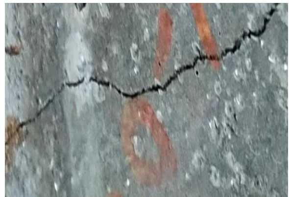
Fig 6: crack developed at third stage of loading
