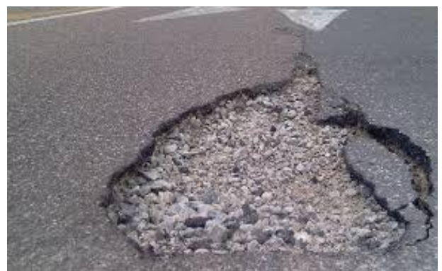
Fig. 1 Water filled and dry road Potholes
