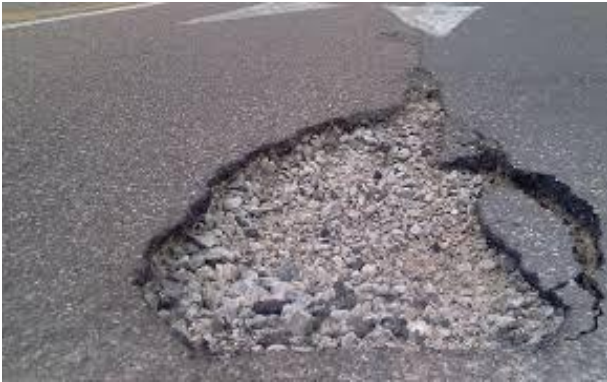
Fig. 1 Water filled and dry road Potholes
