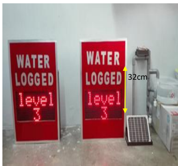
Fig. 11 When the water level is at the third level
