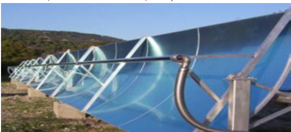
Figure (4) Parabolic Trough Solar Collector (PTC)
