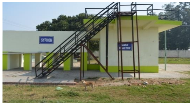
Figure 2: View of UASB Reactor at SWINGS WWTP, AMU Aligarh
