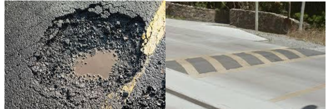
Fig. 1 Potholes and Humps on Roads
