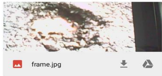
Fig. 15 Pothole detected and sent to BMC through e-mail
