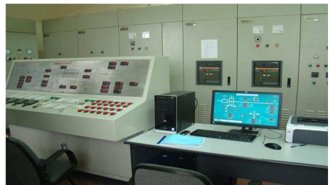
Fig. 12 SCADA center for monitoring and controlling the main pump station
