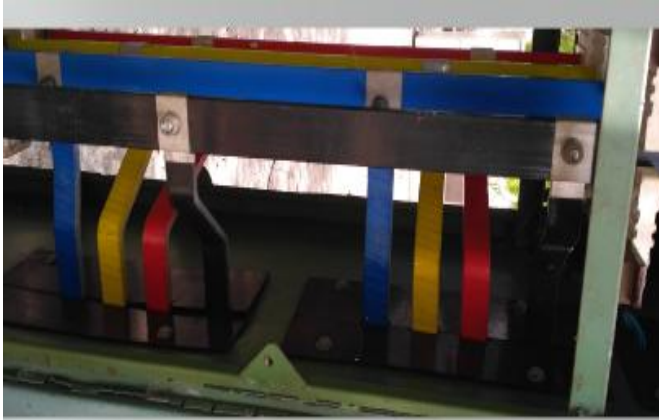
Fig.2 Bus bar panel arrangement in the power house
