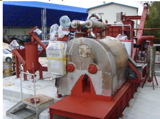
Fig. 6. Batch type high speed drying device connected with vertical pyrolysis combustion device
