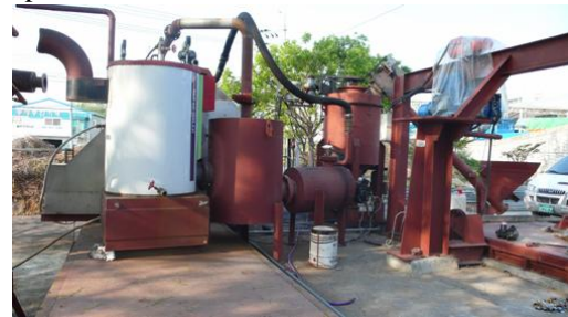
Fig. 5. Vertical Pyrolysis Combustor and Steam Boiler
