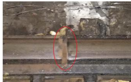
Fig 4.1 Crack On Railway Track
