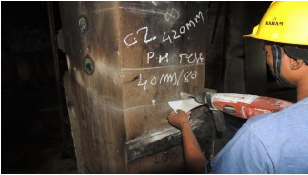
Fig. 4. pH and Carbonation Test
