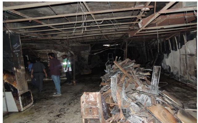
Fig. 1. Fire damaged basement
