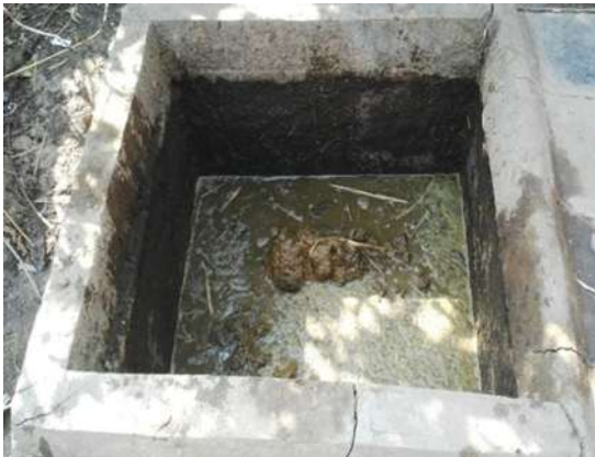
Figure 3: feeding of organic waste in inlet chamber
