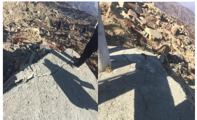
Fig.4 Damaged Platform of T-15 (between Station-G4 and G3)
