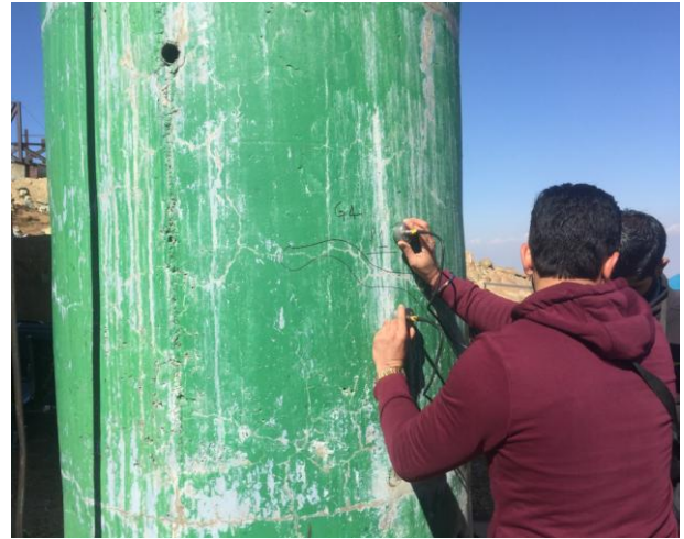
Fig.3. Testing of Column using Ultrasonic Pulse velocity test to check the crack depth
