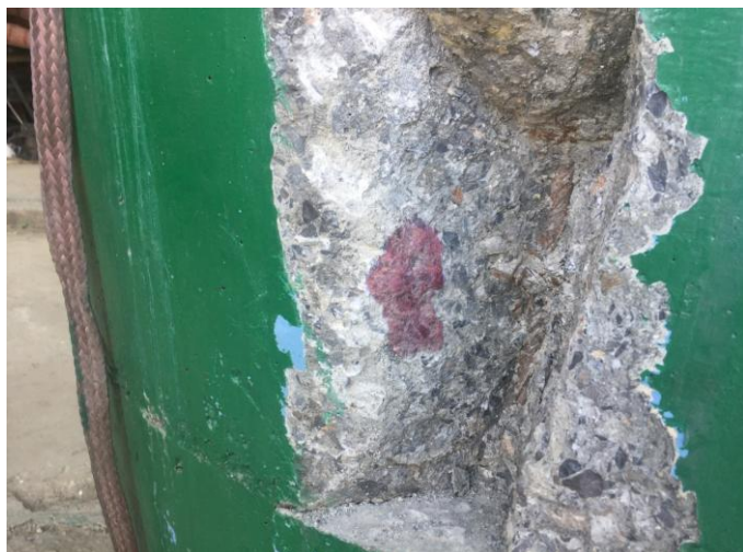
Fig.6 In column P2 of Station G-1 the Column is damaged and on carbonation test showing red colour confirming the carbonation of concrete
