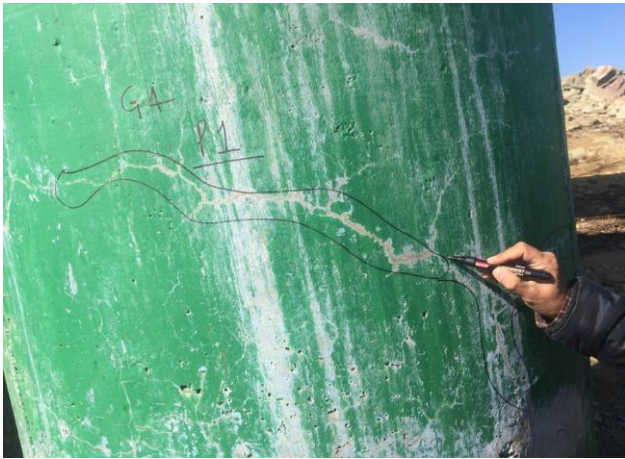
Fig.1. Superficial cracks on Column P1 of Station G-4
