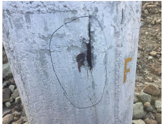
Fig.5 Column of tower T7 had very less concrete cover, reinforcement bar is visible and rusting of reinforcement has been initiated
