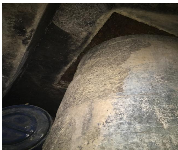
Fig.8 Outer surface of column P6 of station G-2 was observed to be abrade by the materials stored in the store room. No paint/protective coating was done on this
