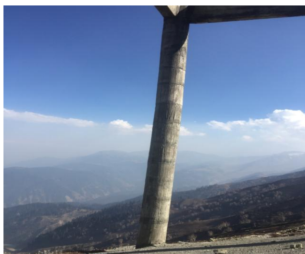
Fig.7 Downhill column of Tower T12 (between G-4 and G-3) was observed to be out of plumb
