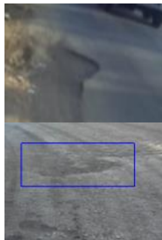
Fig. 7: Images of Potholes A and E
