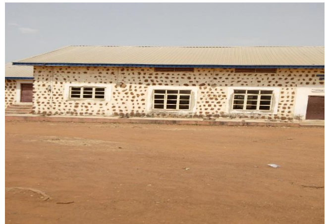
Fig. 3. Stone materials used for walling in Offa Grammar School Hall, Kwara State Nigeria. Built-in 1943.
