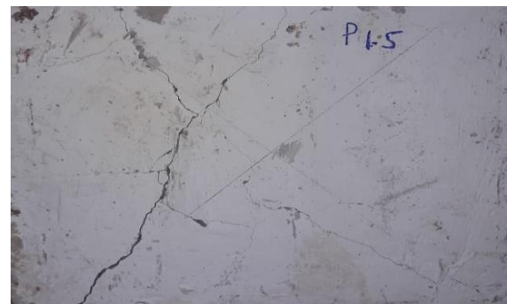
Fig 10:Crack Pattern of FRCP (CT) 1.5% Fiber Content Slab
