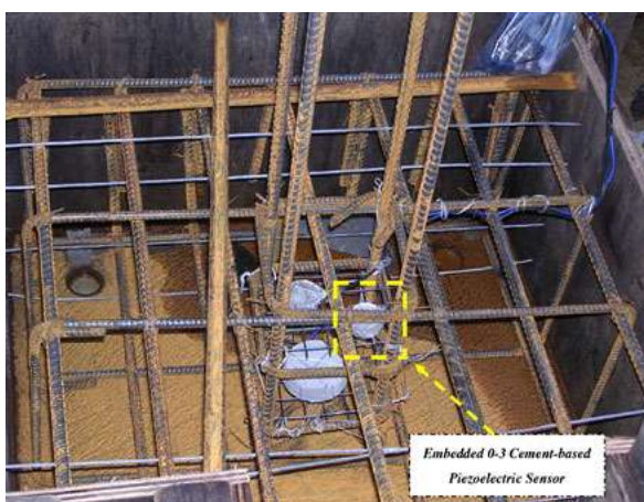
Fig.6: Installed Cement-Based Piezoelectric Sensor
