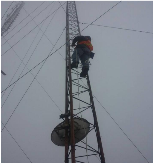
Fig. 6: Tower in Villonaco Hill
