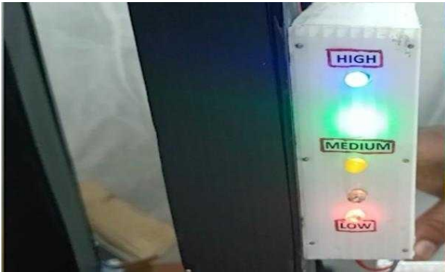
Fig. 7: LED showing water level
